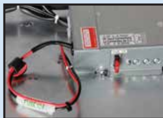
Connection cable with fuse
